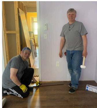
Volunteers Paul Roy and Wilson Velasquez lay the new floor. Paul also served as the project manager for the renovation.
